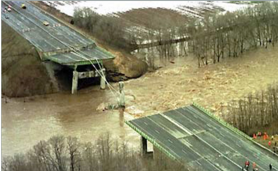
Figure 3.27 View of the Schoharie Bridge after its April 1987 failure due to scour
