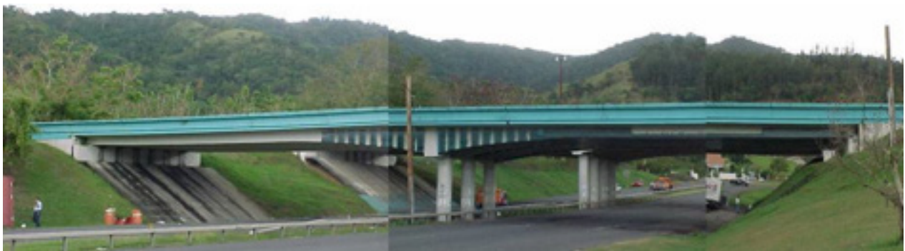
Figure 2-23 Elevation of a bridge that has had CFRP strips added to increase the reinforced concrete’s shear strength
