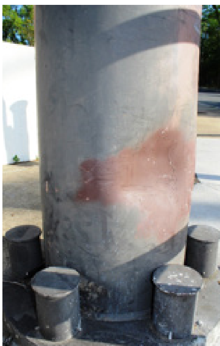
Figure 2-35 An impact-damaged metal pole
