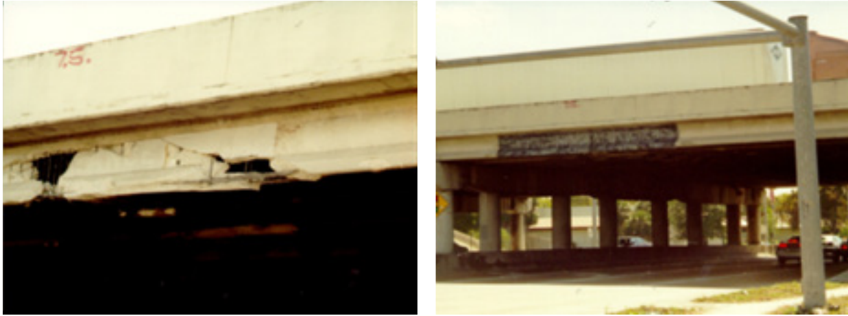
Figure 2-1 An impact-damaged bridge before (left) and after (right) being repaired with bonded CFRP
