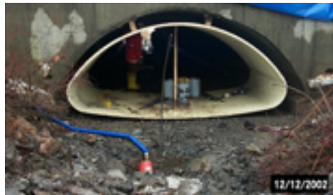
Figure 2-32 Prefabricated FRP arch sections can be slid into an existing culvert, then grout added between them to transfer load to the FRP
