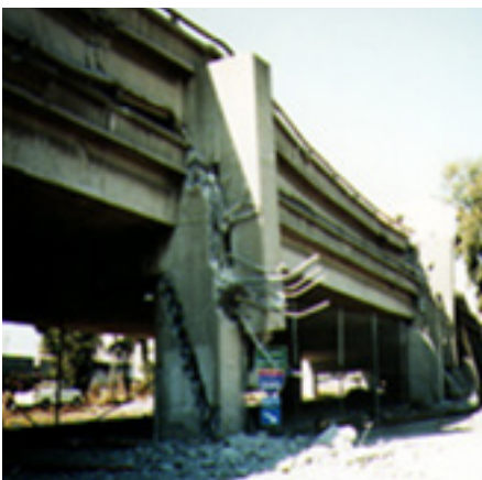
Figure 2-14 Shear failure of a concrete bent due to seismic loading
