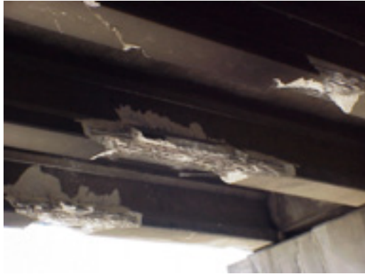
Figure 2-2 Impact-damaged P/S girders
