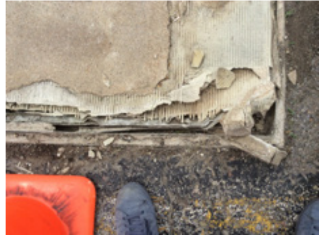
Figure 2-50 Close up of deteriorated utility box cover
