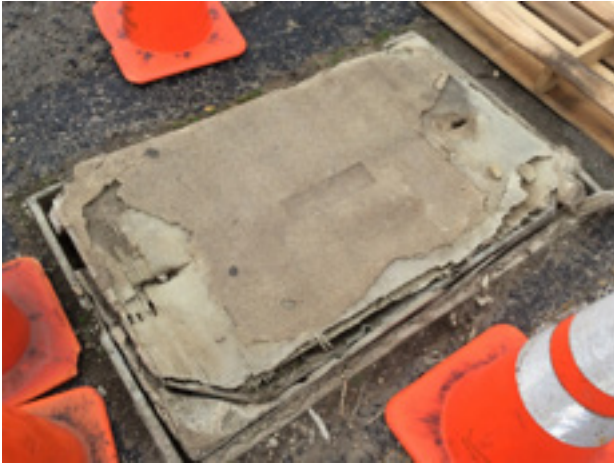
Figure 2-49 GFRP utility box cover in poor condition
