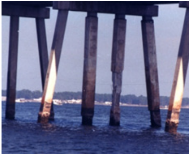
Figure 2-19 Concrete bent damaged by exposure to salt water
