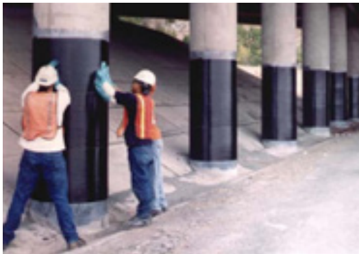
Figure 2-17 Wrapping round concrete columns with CFRP to improve seismic performance by providing additional confinement
