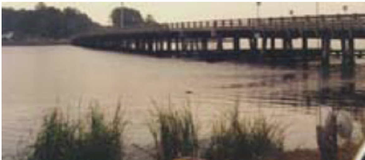
Figure 2-10 Elevation view of bridge in proximity to salt water (Brown's Creek, Jacksonville, FL)
