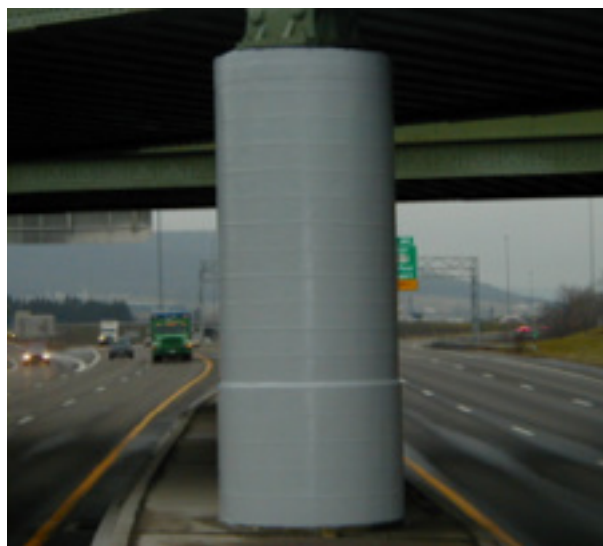
Figure 2-21 The column shown in Figure 2-20 after repair and protective wrapping with GFRP
