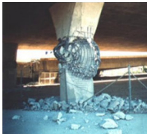
Figure 2-15 Primary steel, buckled during an earthquake due to insufficient lateral confinement
