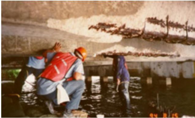
Figure 2-8 Corrosion-damaged concrete beams
