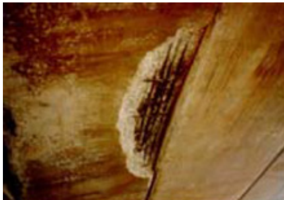
Figure 2-11 Spalled concrete and corroded steel on underside of the bridge shown in Figure 2-10
