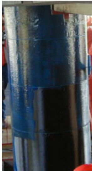
Figure 2-16 Concrete column wrapped with CFRP, prior to application of UV protective coating
