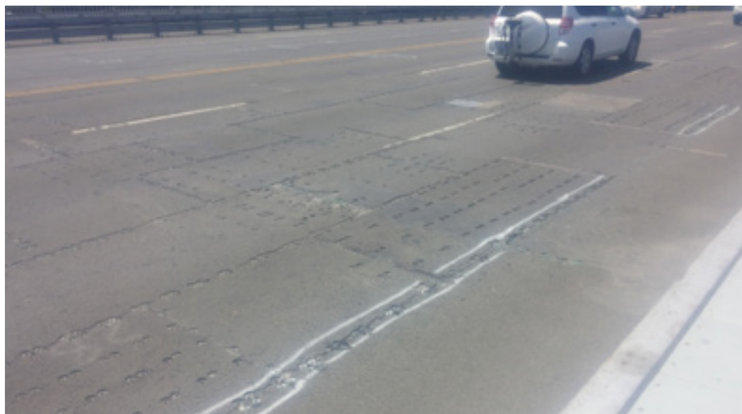
Figure 3-27 Deteriorated and repaired riding surface on the Morrison Bridge Photo courtesy of Multnomah County Public Works Programs 57
