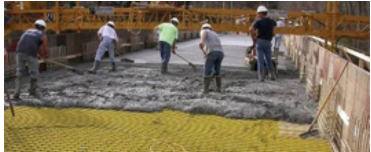
Figure 3-12 Concrete placement on the combined reinforcing/SIP form product shown in the previous figure.
