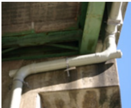
Figure 3-38 An FRP drain system in Oregon
