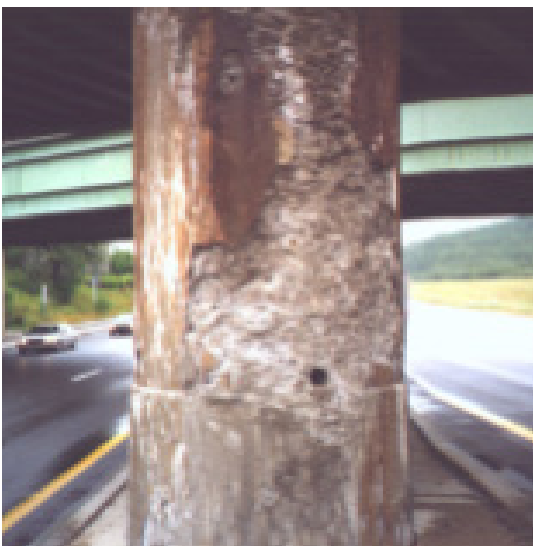
Figure 2-20 A concrete column in the median of a highway that has deteriorated due to salt spray
