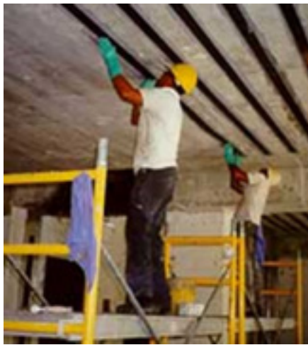
Figure 2-22 Bonding pre-cured CFRP strips to the underside of a concrete slab to increase its flexural capacity
