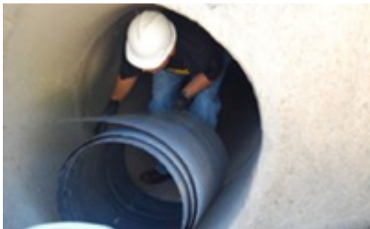
Figure 2-33 One method of relining an existing culvert is to use precured FRP sheets
