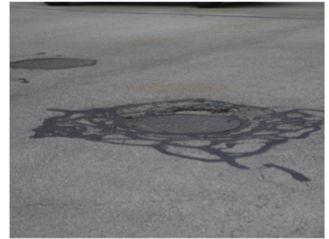
Figure 2.4 Excess sealant (“tar snakes”) reduces surface friction (photo courtesy of Fran Bents)
