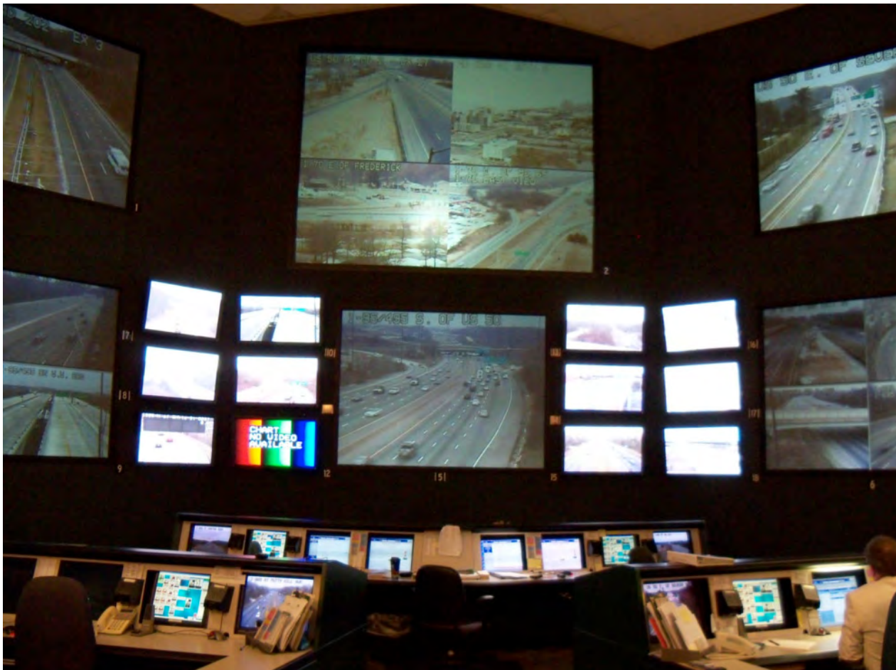
Figure 3.6 Managing incident and work zone traffic impacts at the Maryland DOT TMC
